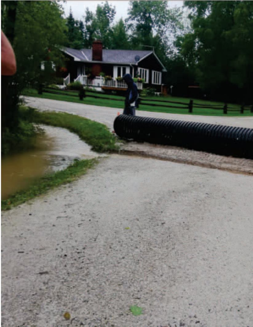
Culvert Blow Out Under Paradise Bay Road August 2022
