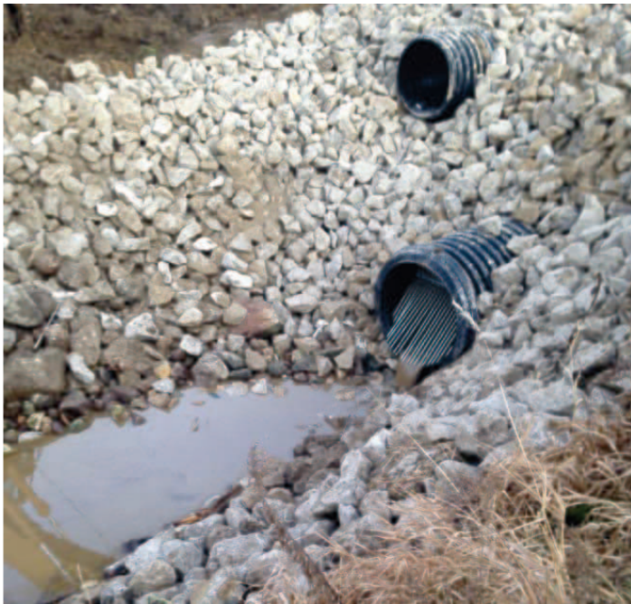
Example of the outlet of a closed Municipal Drainage System
