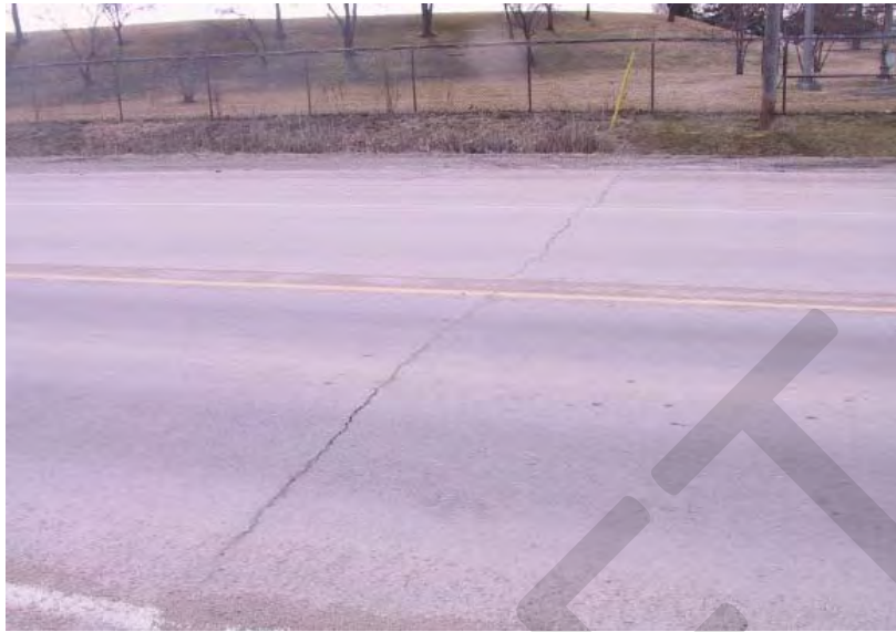
Transverse /Thermal cracking
