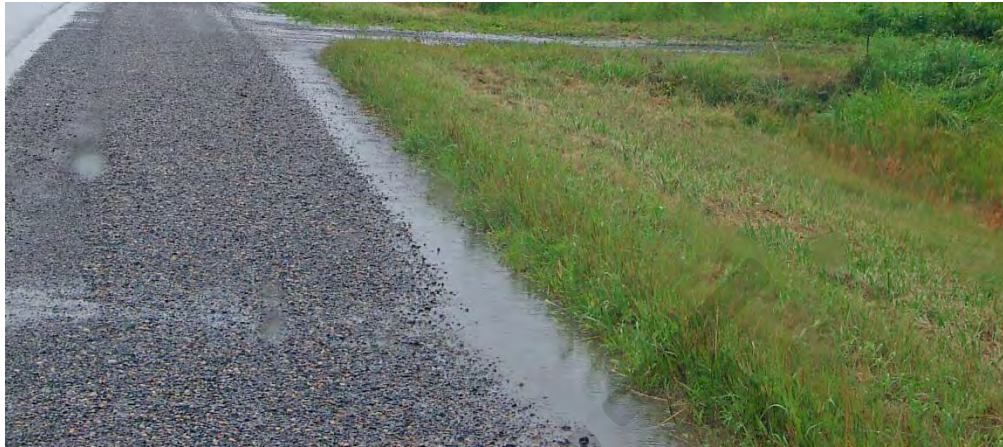
Figure 3.4: Poor Shoulder Drainage (example)
