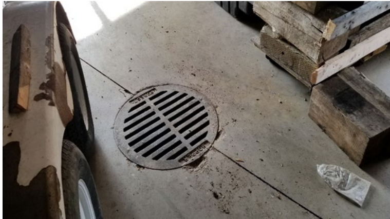
Photo 11 – Floor drain noted in the center portion of the garage in Building B.
