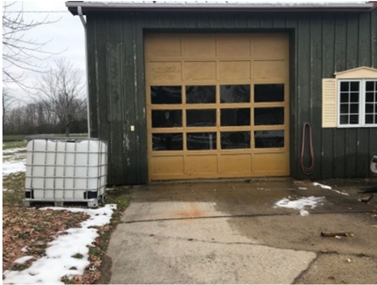
Photo 9 – View of Building B. facing east. Note: brown staining on concrete and empty storage tank.
