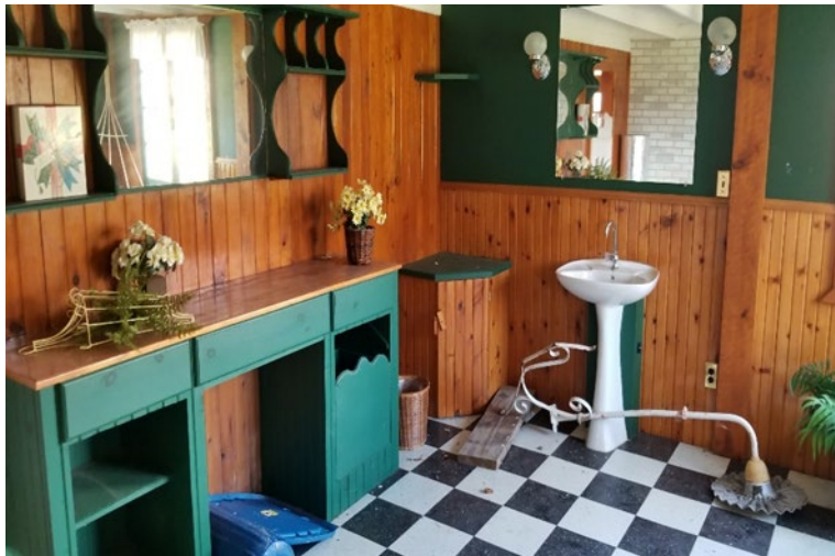
Photo 12 – Interior view of Building B. Note: potential vinyl floor tiles containing asbestos.
