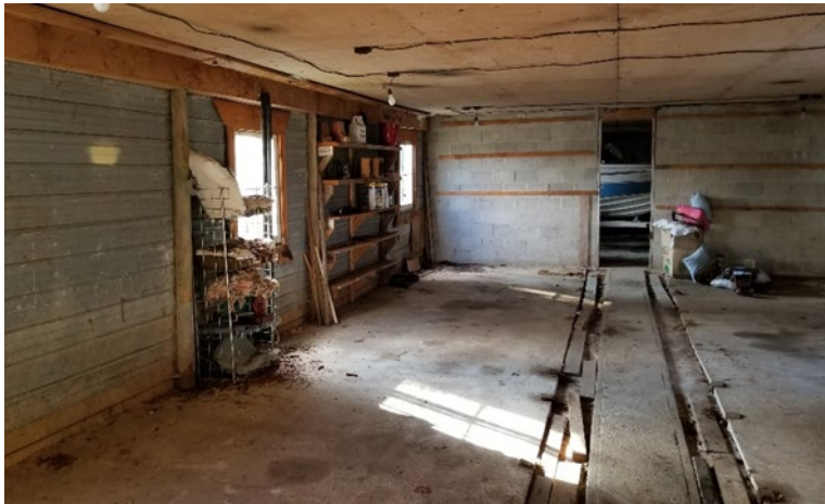
Photo 15—Interior view of Building C. Note: cracked concrete and staining.
