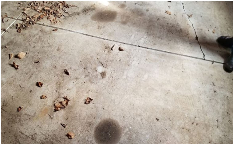
Photo 20 – Interior view of Building E. Note: cracked concrete and staining.
