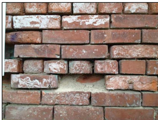
The loss of mortar can cause damage to brick buildings. Mortar should be re-pointed when it begins to deteriorate.
