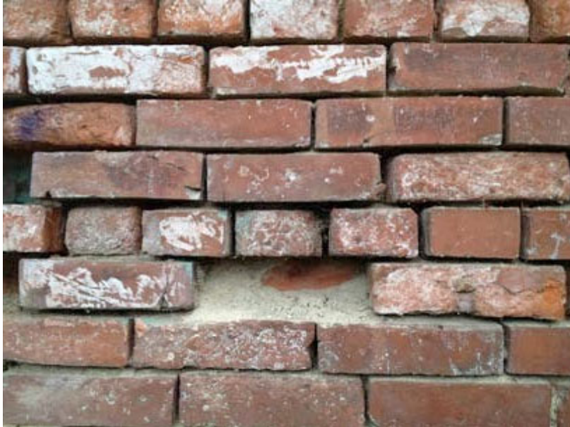
Figure 7: Example of Loss of Mortar in Brick
