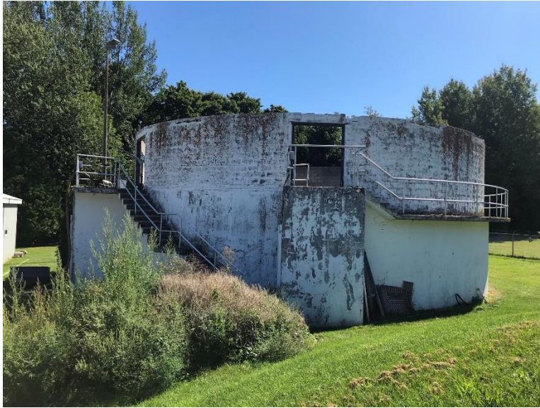
Figure 17: Digester, not in service (A.S.I. 2022)
