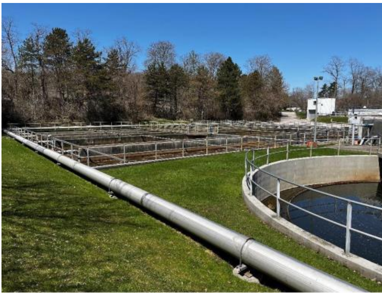
Figure 29: Infrastructure in the Paris Water Pollution Control Plant (A.S.I., 2022).
