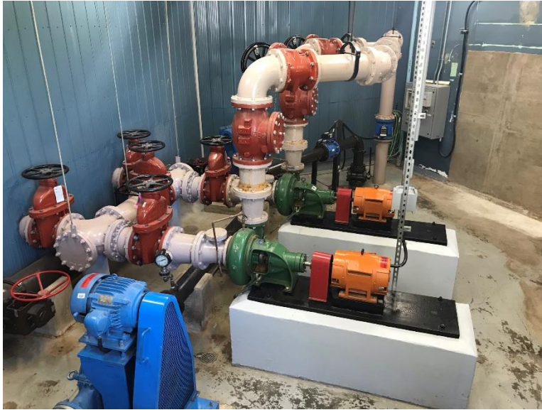
Figure 19: Representative waste water pumps (A.S.I. 2022)
