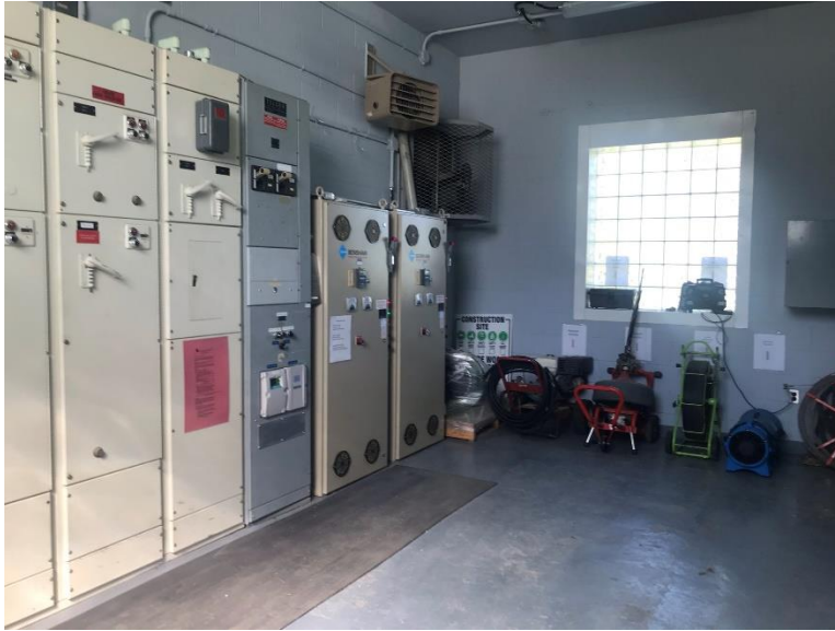
Figure 11: Electrical controls in the pumping station (A.S.I. 2022)
