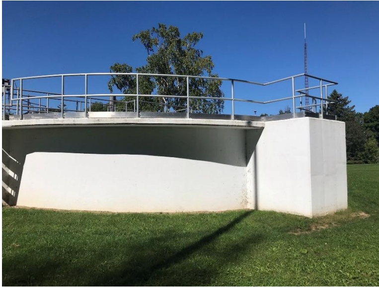
Figure 15: Secondary clarifier (A.S.I. 2022)
