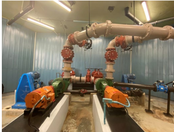
Figure 7 – RAS and WAS Pumps
