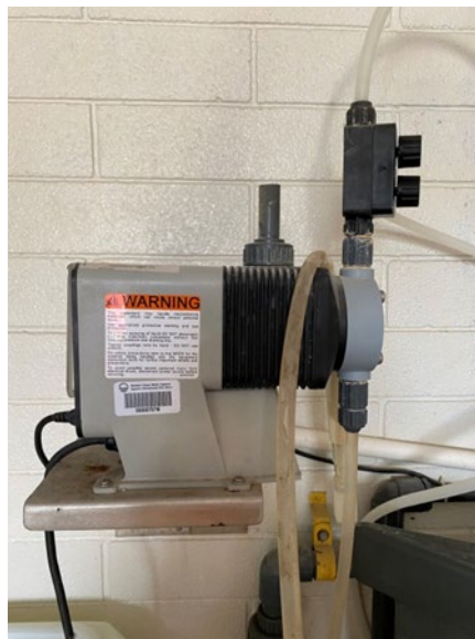
Figure 9 – Sodium Hypochlorite Chemical Dosing Pump
