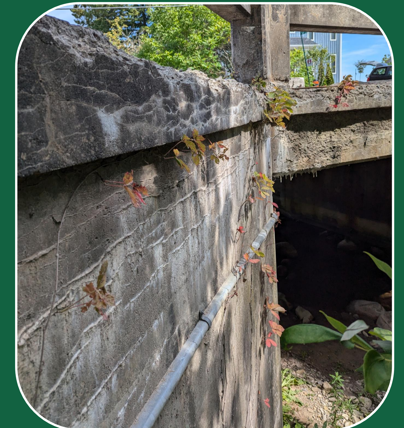
Delamination and Cracking on Wingwalls
