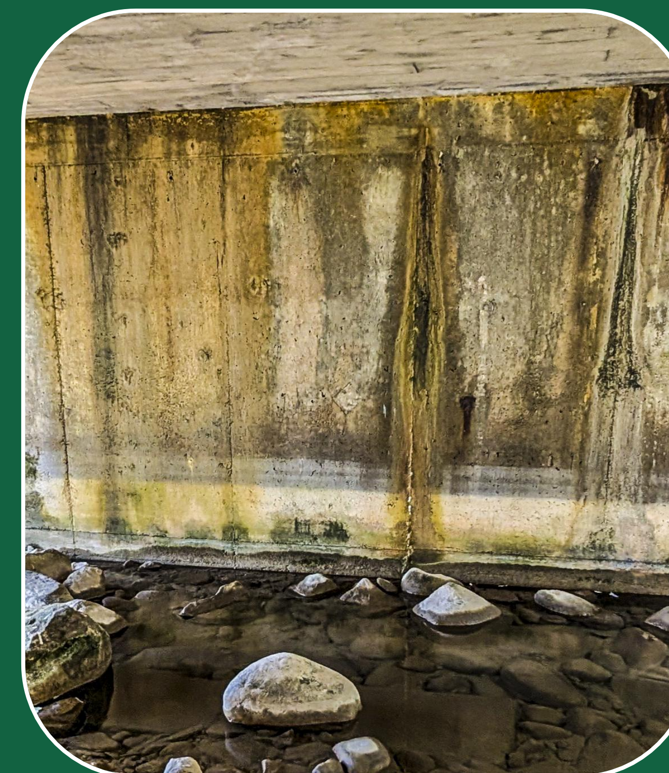
Water Infiltration Through Abutments
