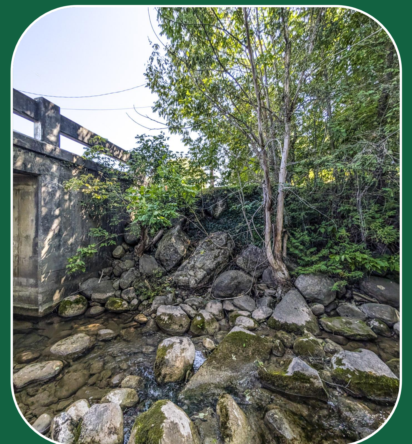
Steep and unstable Embankments
