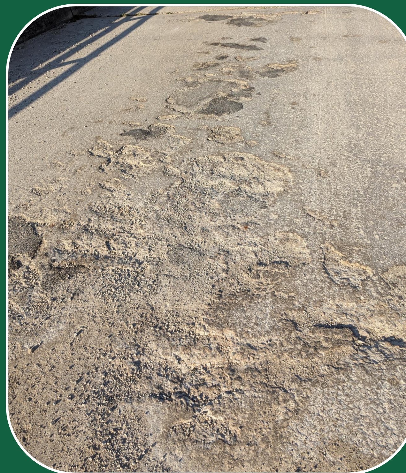
Concrete Spalling on Deck
