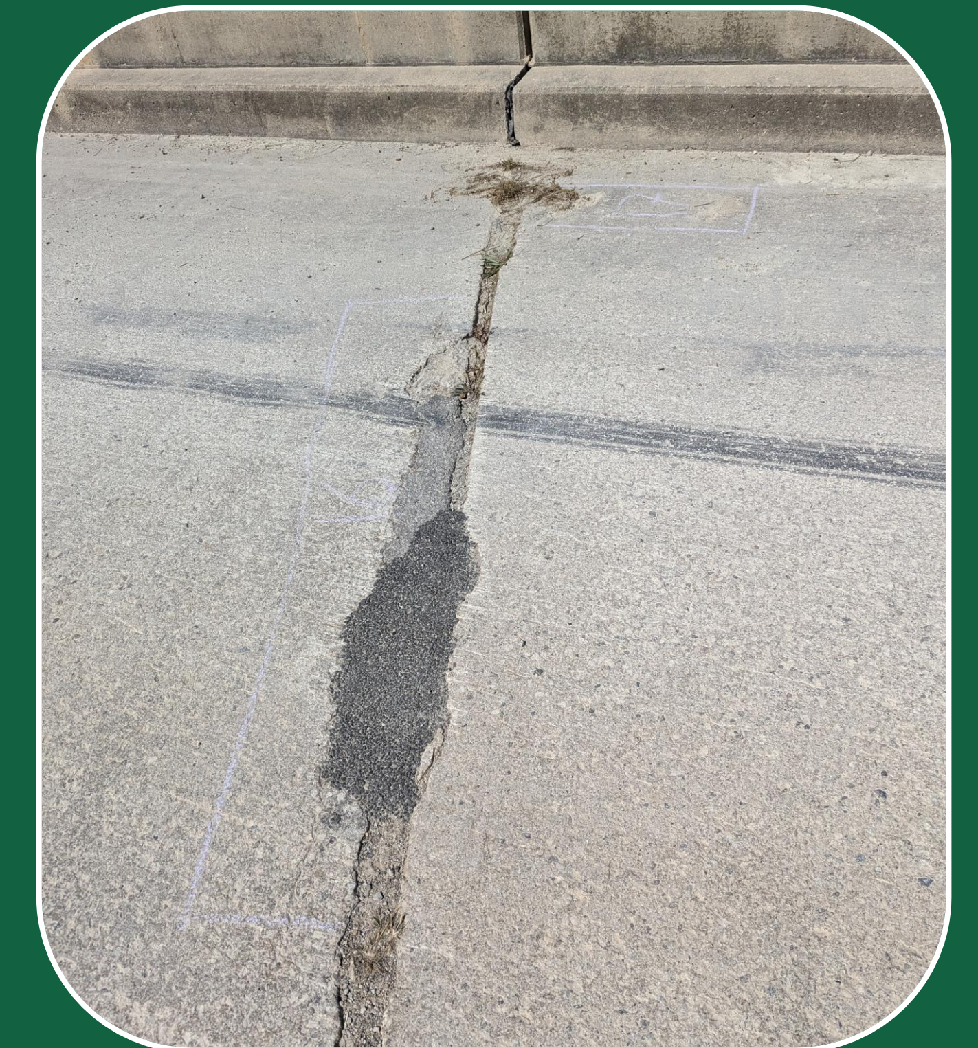
Patchwork in Expansion Joint
