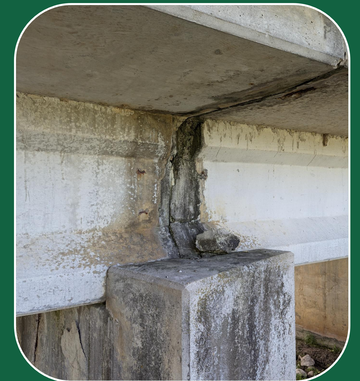
Deterioration in Expansion Joint
