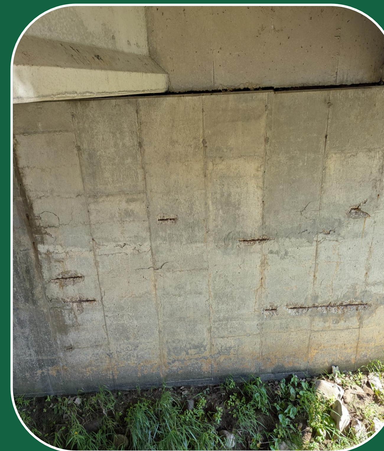
Exposed Rebar in Abutment
