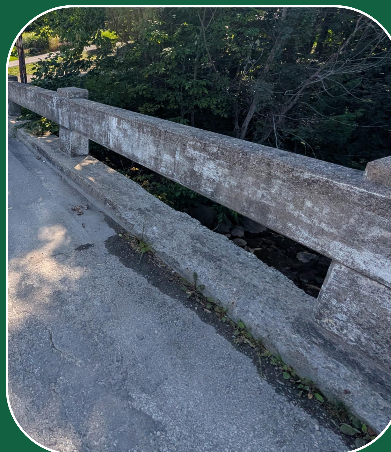
Typical Deterioration at Concrete Curb
